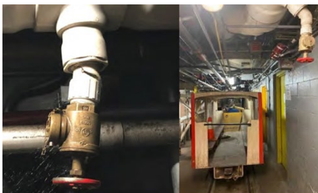
Cracked Low Point Drain
