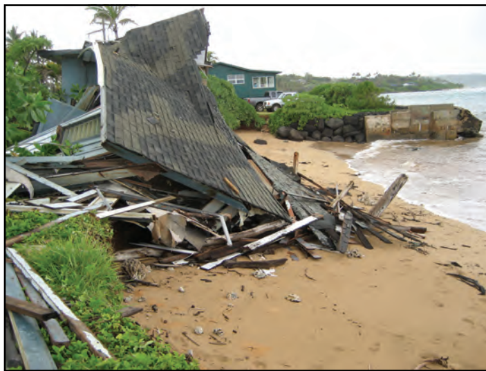
A seawall built on property adjacent to this house at Aliomanu Beach is cited as a likely cause for the severe erosion of 100+ feet of land seaward that led to its gradual and eventual collapse that necessitated owners demolishing it in April.
