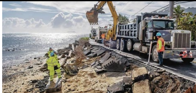
Kuhio Highway at Wailua Beach is on the verge of requiring emergency repairs similar to Kamehameha Highway on Oahu. Climate change-driven sea level rise and erosion damage prompted emergency repairs on Feb. 11 to address high surf impact near Swanzy Beach Park in Kaaawa. Photo: Dennis Oda, Star-Advertiser
